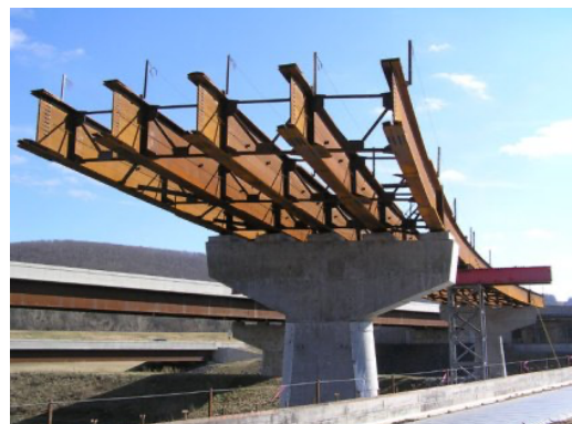
Steel I-beams in bridge construction showing the vertical web sandwiched between top and bottom horizontal flanges
