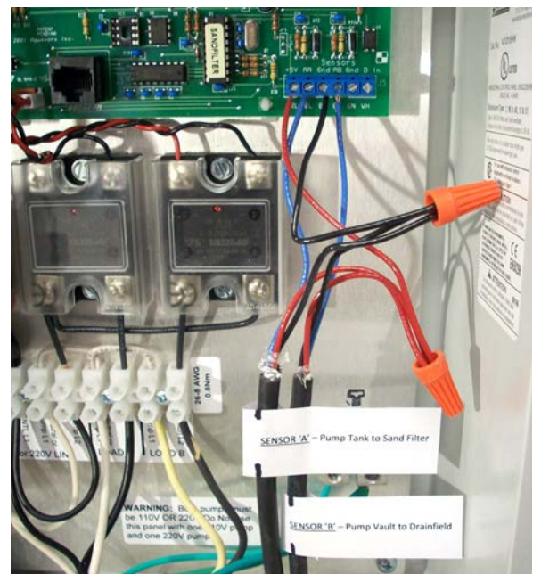
Figure 8: Sand Filter Panel
