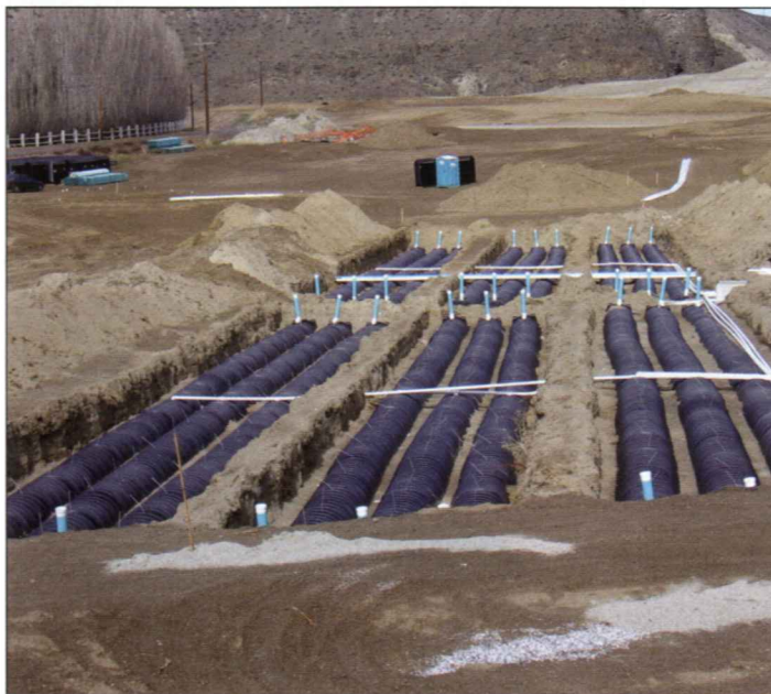
A community cluster system at Crescent Bar, a resort community in Quincy, Washington. Image: Infiltrator
