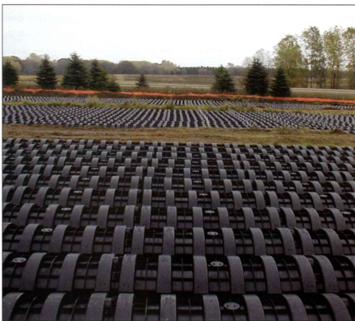
The Fields of St Croix wetland system being installed at Lake Elmo, Minnesota. Image: Infiltrator
