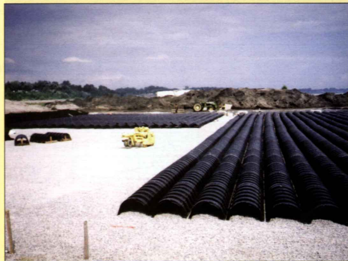
The installation of chambers at the Port Burwell Sewage Treatment Plant in Ontario. Image: Infiltrator
