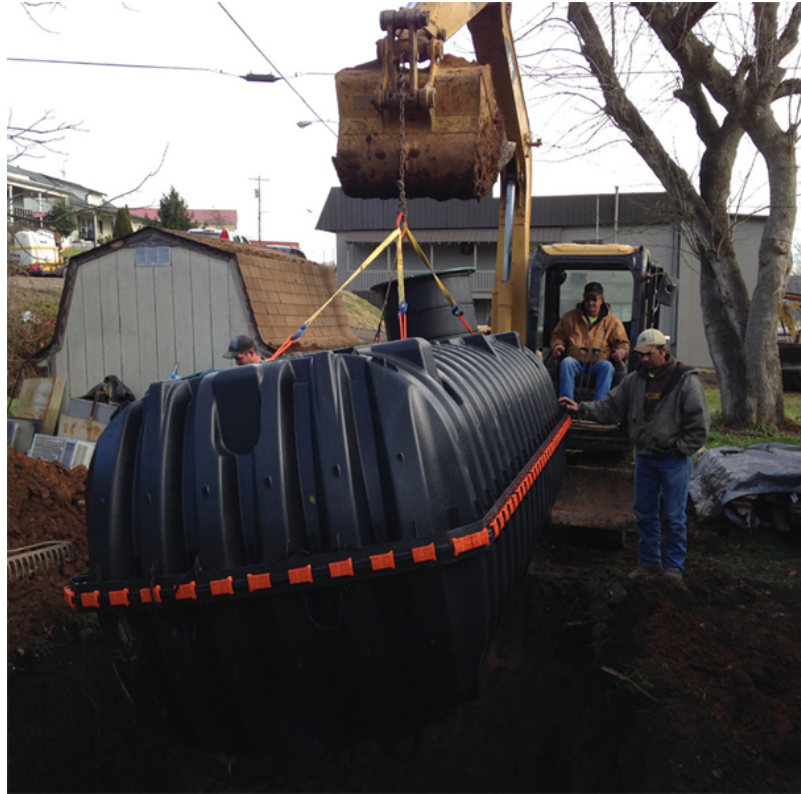
At Surgoinsville, TN, the difficult Appalachian sites with steep slopes and limited backyard access to existing homes made system design and installation challenging. Ultimately, individual STEP services were installed at more than 200 residences. The ease of handling the plastic tanks in tight quarters made them the ideal solution.
