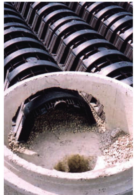
The Port Burwell Sewage Treatment Plant uses Infiltrator chamber technology in an exfiltration bed instead of an outfall as a discharge solution. Photo by Infiltrator Water Technologies
